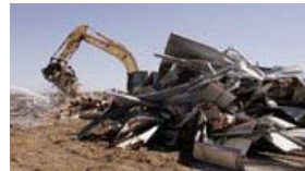
Cranes yesterday pulled apart the apartment buildings, which were constructed of all-metal framing.
